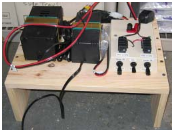
Inverter, Battery Charger, Switchbox, Shelf (Charger On-Off, AC-Battery, Inverter On-Off)
