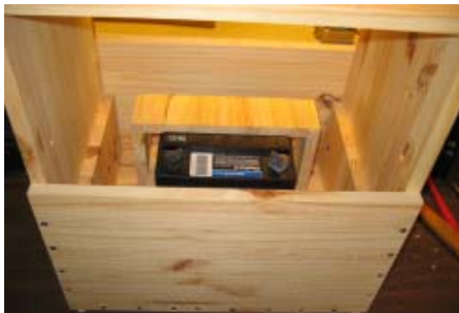
Battery inside the Battery Module
